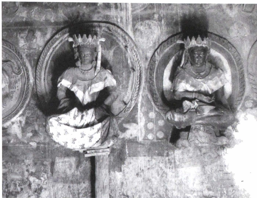
Fig. 11. The section of the Tabo Assembly Hall damaged in 1837. The restoration is recorded in an inscription on paper attached to the wall Main Temple, Assembly Hall, north wall
